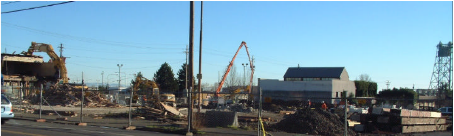
Concrete was poured this afternoon for Vancouver hotel-convention center, beating construction deadline by 13 days. Building at the left is old Greyhound Bus Station being demolished. Webber Machine building is in background, Interstate Bridge Tower, right.
