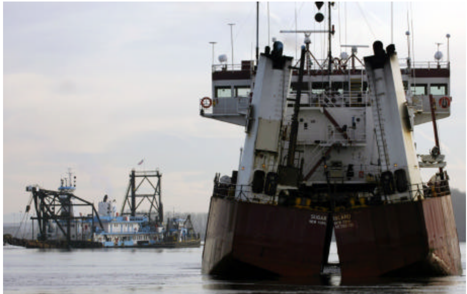
Dredges Sugar Island, foreground, and Oregon, left, have completed over one-quarter of the Columbia River channel deepening project, increasing depth of the river to 43 feet from Vancouver west about 25 miles and a smaller section of the river east of Astoria. The pipeline dredge Oregon, owned by the Port of Portland ‘rehandled’ 2.6 million cubic yards of sand, depositing it on industrial sites at the Ports of Vancouver and Portland.
